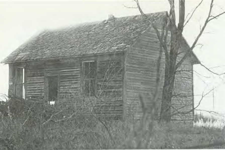
This empty shell is all that remains of the first real school in the Merino area. The Southside School, built in 1888 on land donated by Jimmy Chambers, was located at South Platte, the oldest community in present-day Logan County.
